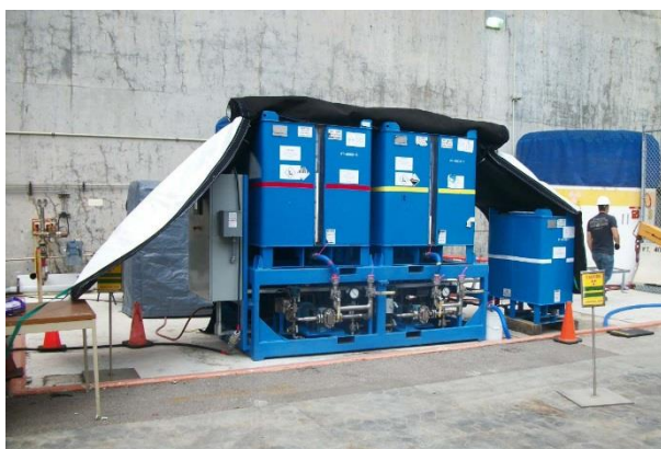
APST TM Mobile Metered Injection System - Primary Resin Solidification at the US Diablo Canyon Nuclear Power Plant
