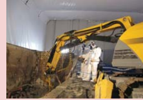
Plant Operations using remotely-operated tools: Utilisation of the BROKK 150C with a Pecker Attachment for Decommissioning activities.
