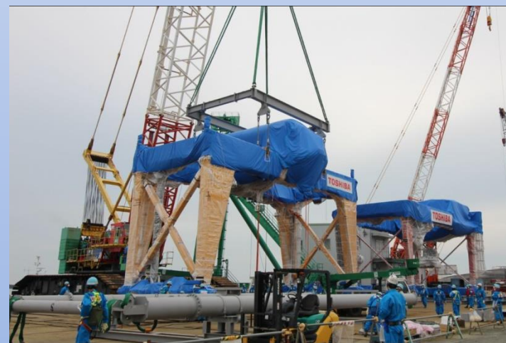
Fuel handling crane and machine
