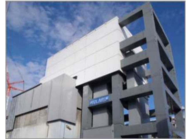
November 12, 2013: Completion of fuel removal facility (The volume of steel used is equivalent to those of Tokyo Tower)
