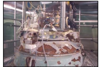
CIRCE - Radioactive liquid tank
