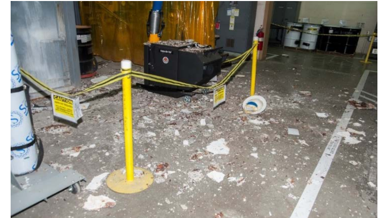
Debris From Ceiling Fall in Y-12 Building 9204-2
